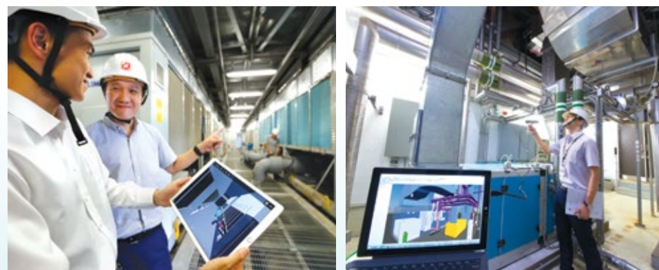
「建築信息模擬—資產管理」系統以立體圖像顯示建築物結構，提高建築物內機電設施的維修保養效率 The Building Information Modelling-Asset Management System provides 3D models of building structures for enhancing the maintenance efficiency of E&M facilities in buildings
