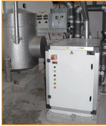
(One heat pump with a 1000L water tank 熱泵及其1000升容量的儲水箱)
