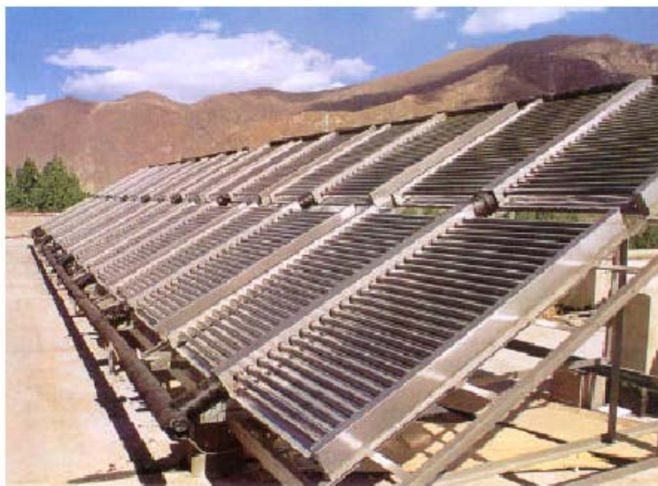
Figure 5-16: Large scale evacuated tube solar collector array
