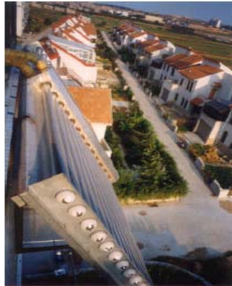
Figure 5-15: Evacuated tube collector mounted on balcony of a high rise building
