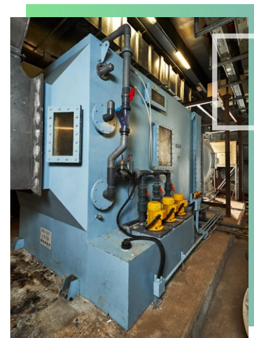
The layout of plant rooms shall be so designed as to allow sufficient space for the installation, operation and maintenance of all plant items
