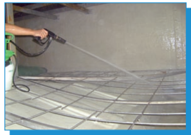
Clean water basin 清洗水盤
