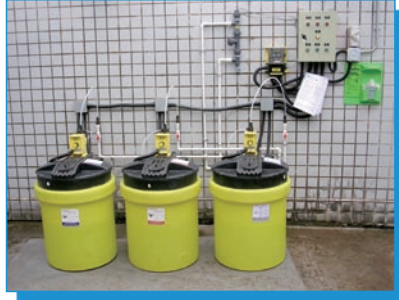
Check conditions of water treatment facilities 檢查水處理投藥設備的狀況
