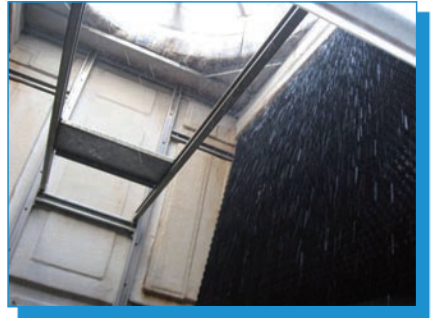
Water showering from drift eliminator 水點由收水器大量瀉出
