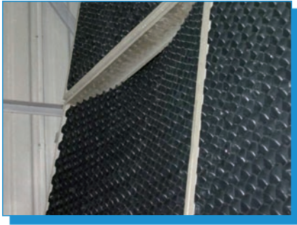
Deformed drift eliminator 已變形的收水器
