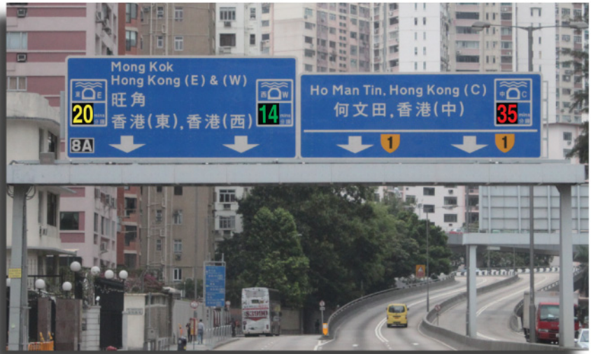
新建立在窩打老道南行近九龍醫院的行車時間顯示器 The Journey Time Indication System newly installed at the south bound section of Waterloo Road near Kowloon Hospital.
