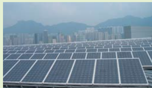
Photovoltaic System at EMSD Headquarters
