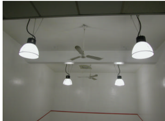
Fig. 12: New induction lighting system
