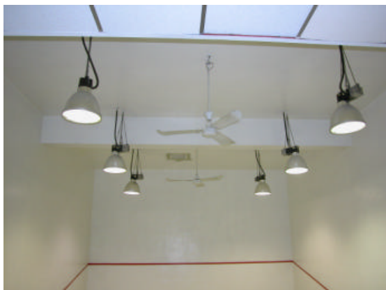
Fig. 11: Existing HID lighting system
