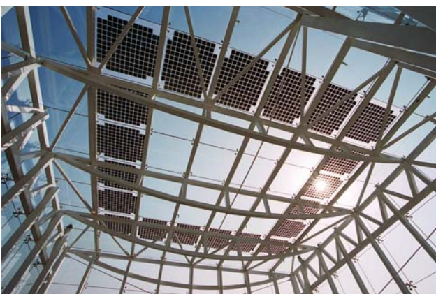
Fig. 2: Photovoltaic glass laminates installed at the Viewing Gallery
