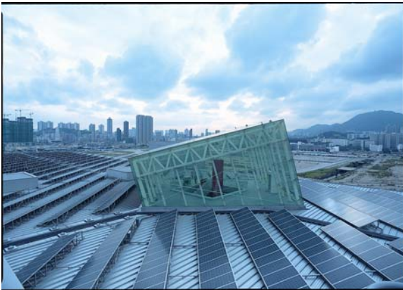
Fig. 1: BIPV installation in EMSD Headquarters
