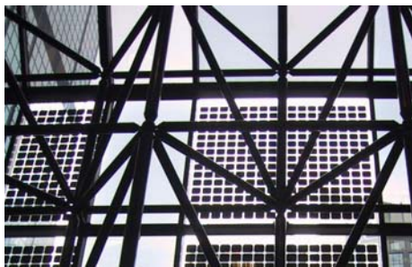
Fig. 7. Skylight Sub-system – Interior view
