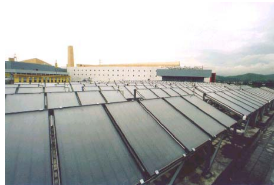
Fig. 1. Solar water heating installation at Sheung Shui Slaughter House
