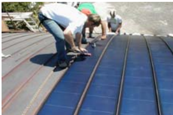
Figure 1: Flexible Amorphous Thin-film PV Panels installed on curved surface (Photo source: NREL)
