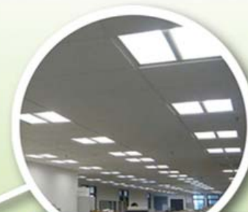
照明裝置 Lighting installation
