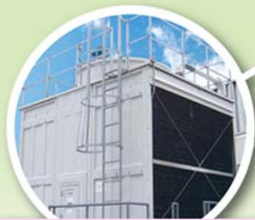
空調裝置 Air-conditioning installation
