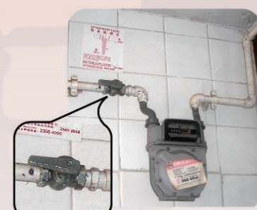
▲ 氣錶前的緊急控制閥 Emergency control valve upstream of gas meter
