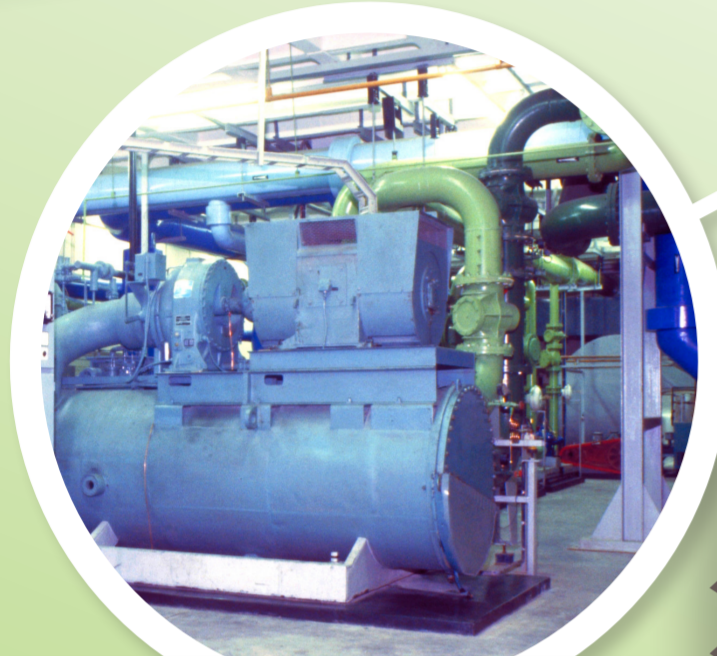
空調裝置 Air-conditioning installation
