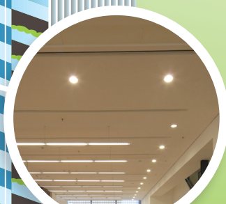
照明裝置 Lighting installation
