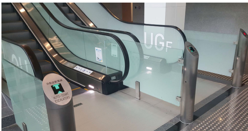
Figure 8.5.7 (a): Example of pole mounted sensors
