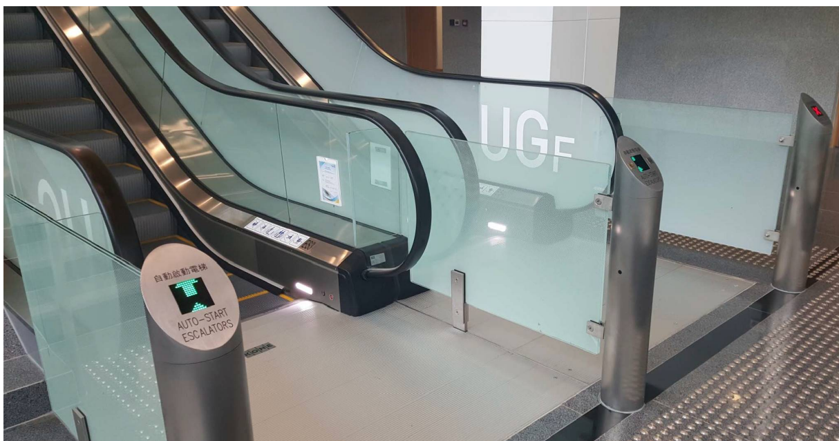
Figure 8.5.7 (a): Example of pole mounted sensors
