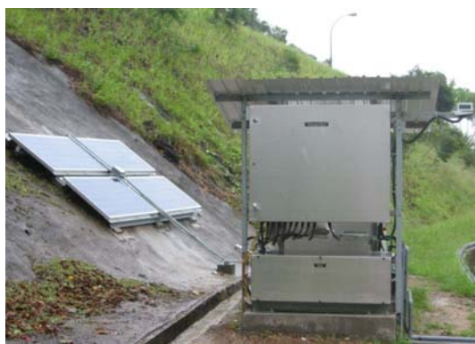
Fig. 3. Automatic Slope Irrigation System
