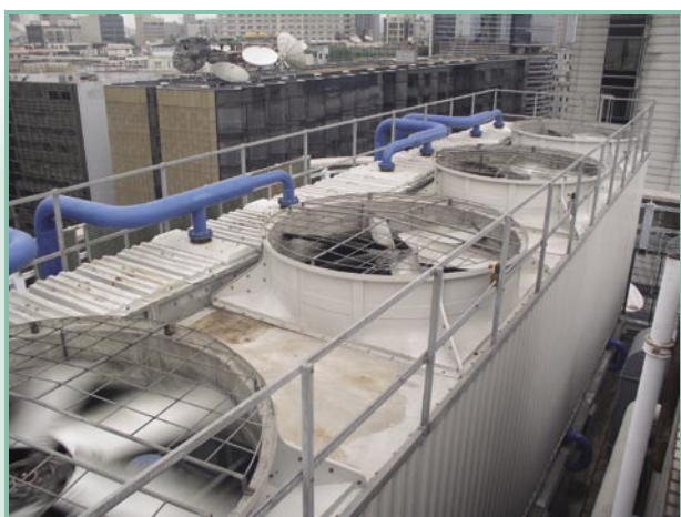
Cooling towers on the roof of the Young Men's Christian Association (YMCA) in Tsim Sha Tsui (cooling capacity: about 1,200 TR)
