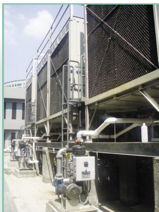
Cooling towers on the roof of the Hong Kong Community College in Hung Hom (cooling capacity: about 2,100 TR)
