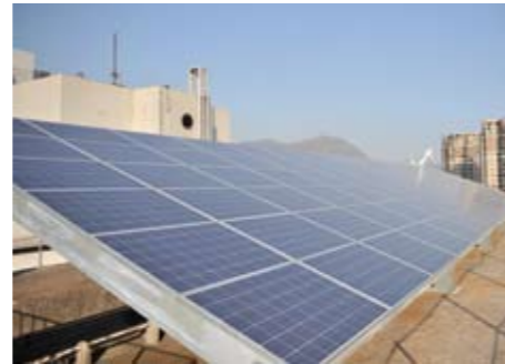
九龍醫院的太陽能及風能混合發電設施 Hybrid Solar Photovoltaic & Wind Turbine System at Kowloon Hospital
