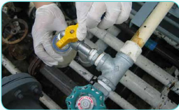
從冷卻塔採集水樣本 Collection of water sample from cooling tower
