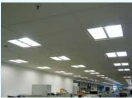
照明裝置 Lighting Installation
