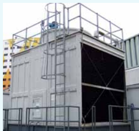
空調裝置 Air-conditioning Installation
