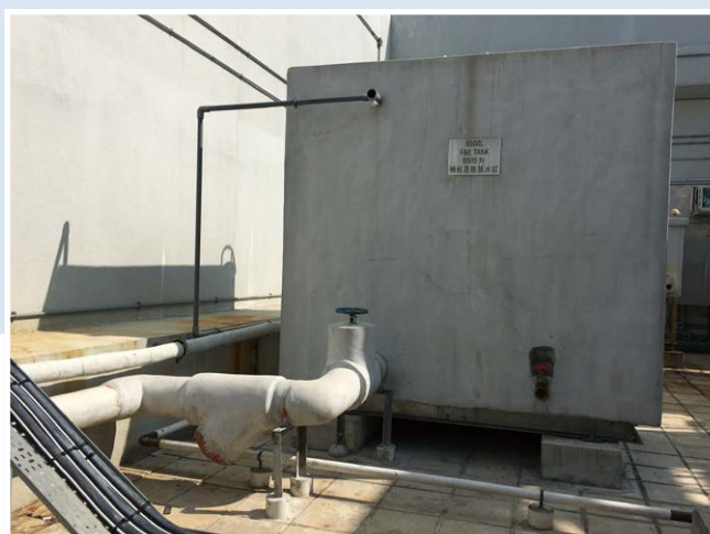
圖5：新大樓的膨脹水箱 Photo 5: The new expansion tank
