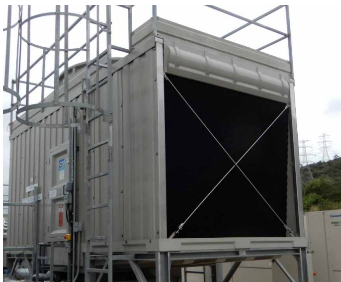
■ 典型冷卻塔 A typical cooling tower
