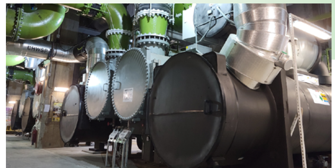
■ 5,000冷噸的製冷機組 The 5,000 tonne of refrigeration chiller
