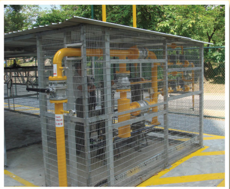
Vaporiser and Gas Main
