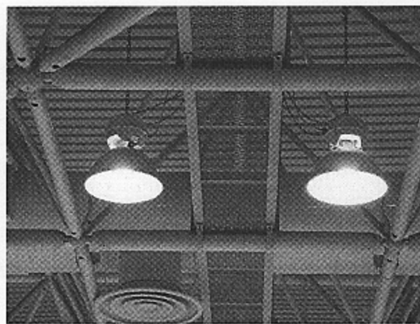
Fig.11: Existing HID lamps and high-bay luminaries at Kowloon Bay Indoor Games Hall
