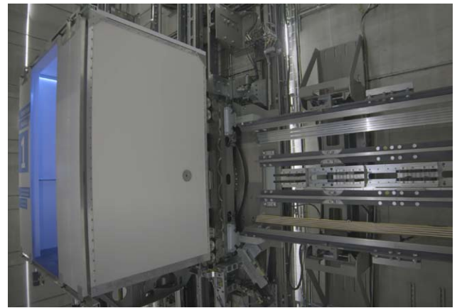
A magnetic levitation lift designed by a German company
