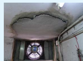
concrete spalling in the lift machine room
