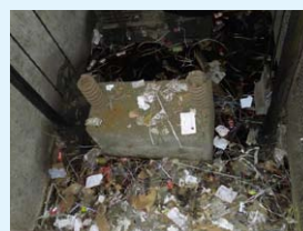
accumulation of waste water or garbage at the bottom of the lift pit
