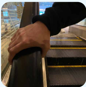
When pulled by hand, the handrail has no slackening
