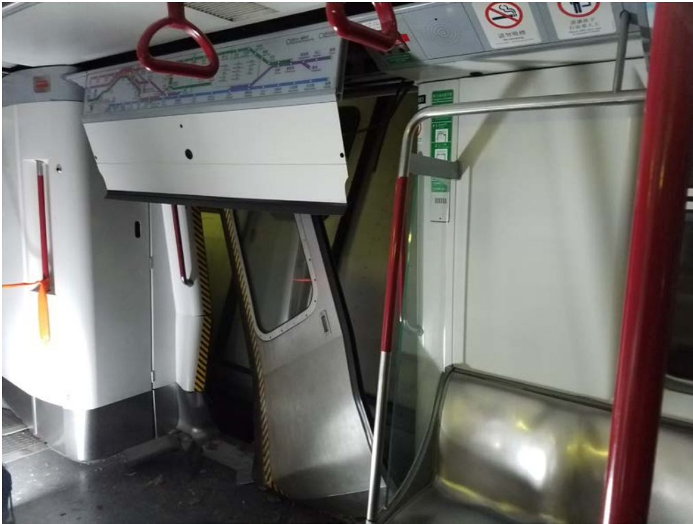
Figure 2: Damage to the saloon of train T112
