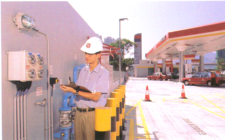
There are over 40 auto-LPG filling stations in service throughout the territory
