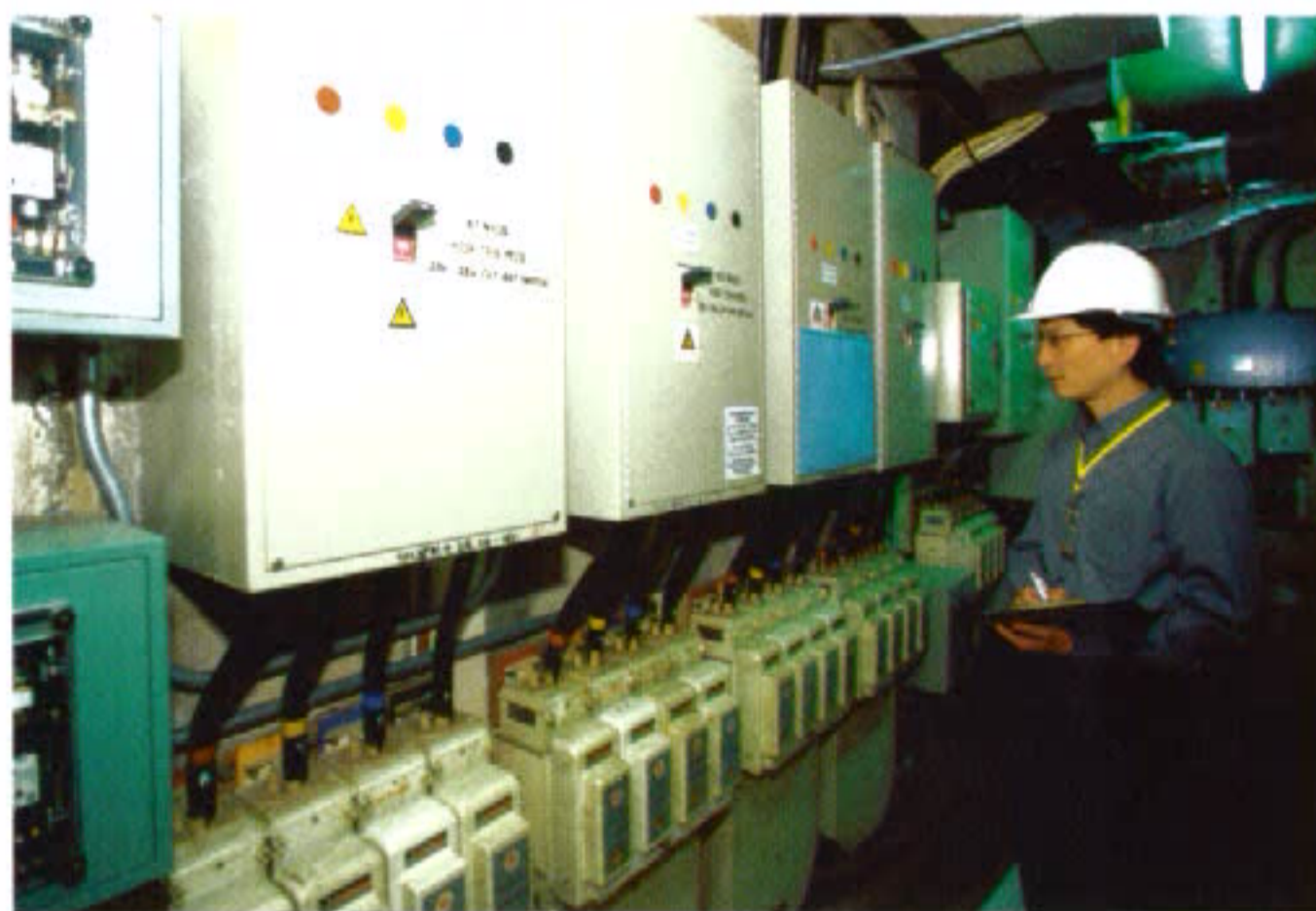
Site inspections are key to ensuring the safety of fixed electrical installations in 2002.
