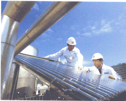
We installed an advanced solar thermal heating system at the Kowloon-Bay Fire Station.
