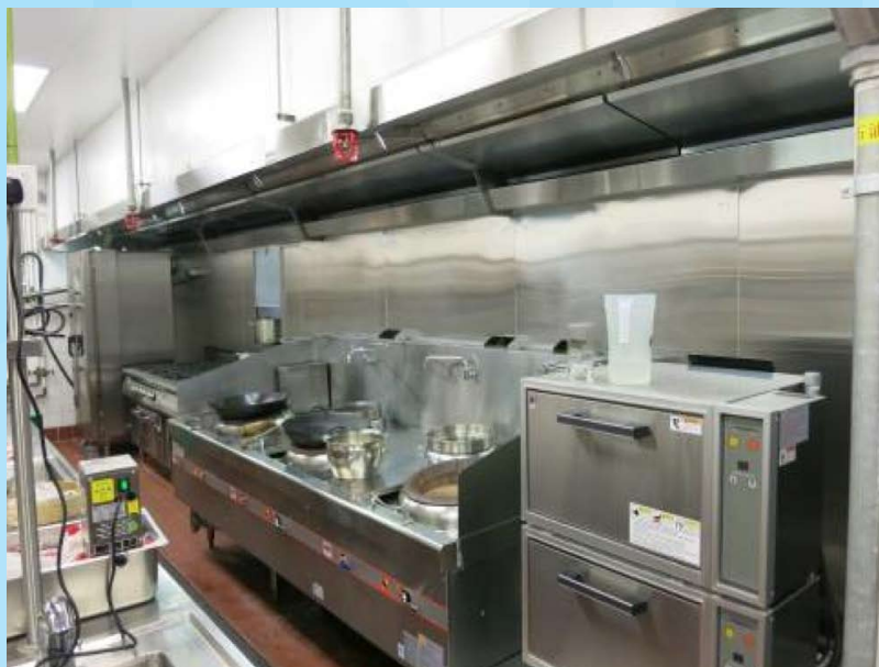
Gas installations in a kitchen
