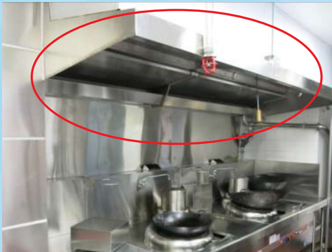
Mechanical Ventilation System
