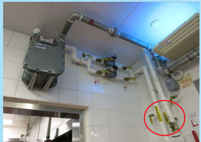
Emergency Control Valve
