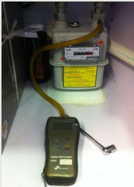
Figure 2: Pneumatic leak test – to gauge the system pressure using an electronic pressure gauge
