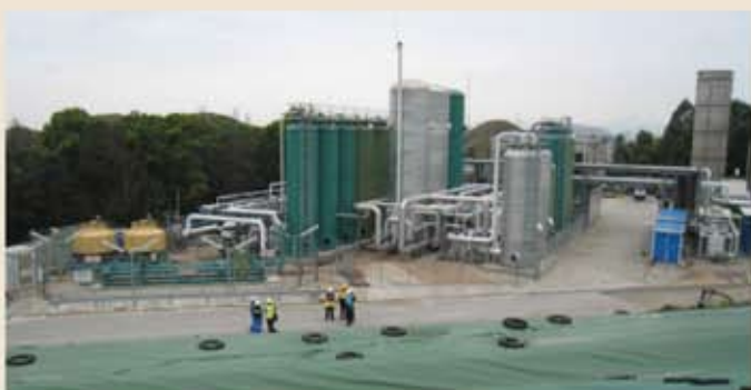
Figure 3 Landfill Gas Treatment Unit at NENT Landfill
