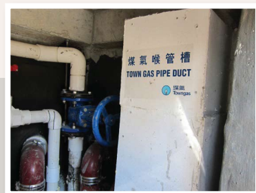
Figure 2: A town gas pipe duct
