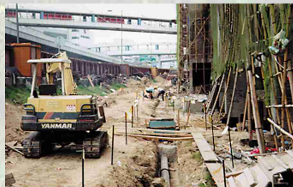
Figure 6: Follow safe excavation practices to ensure that there is an adequate separation distance between any gas pipes and the excavation area.
