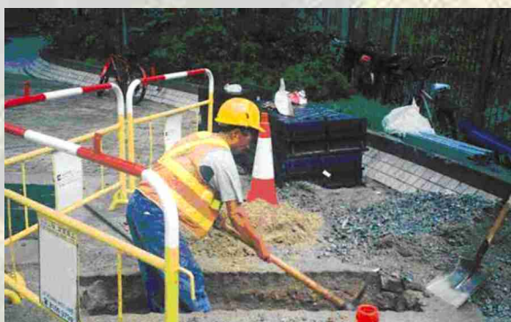
Figure 5: Using hand dug trial holes to confirm the actual location of the gas pipes.
