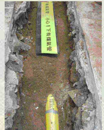
Figure 1: The pipes used to supply gas are laid underneath roads or footpaths.
