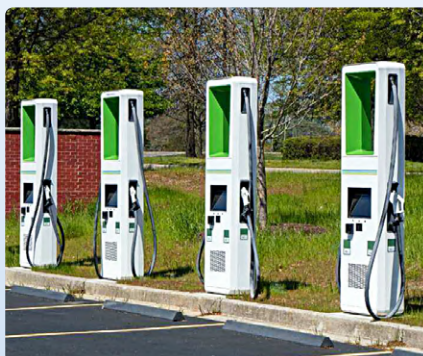
Electric Vehicle Charging Facilities
