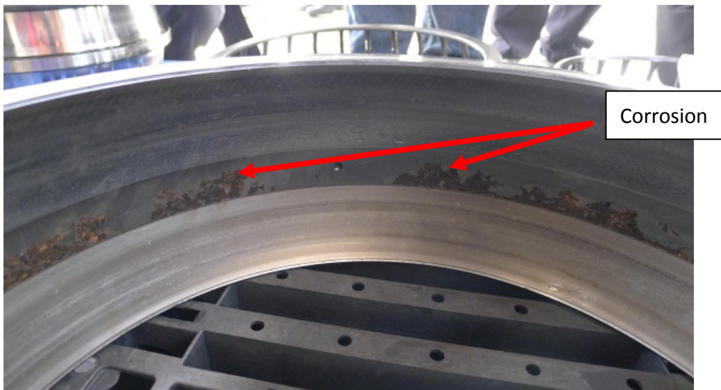
Figure 8: Corrosion in the outer ring of the upper bearing
