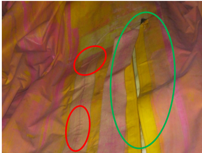
Figure 5b – Some detachments in left covering strip at the centre (circled in red)
