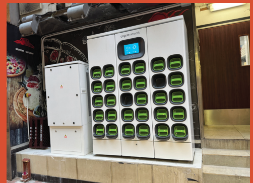
The charging system can charge up to 30 batteries at a time.
