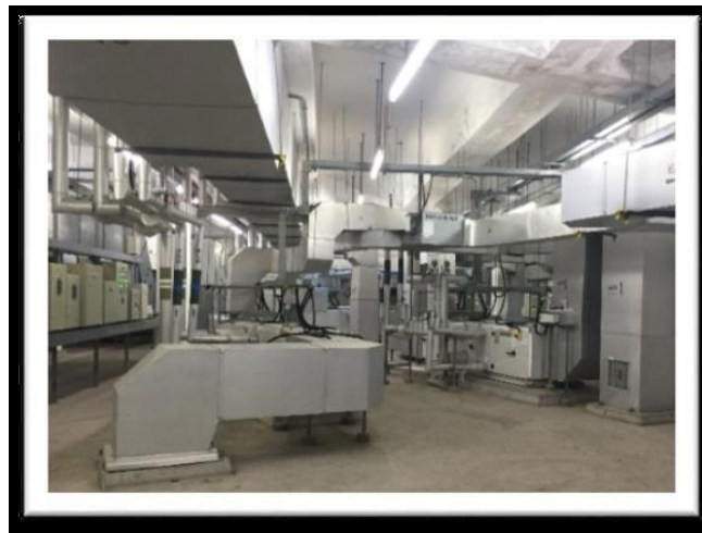
Photo A.8 Air handling unit
