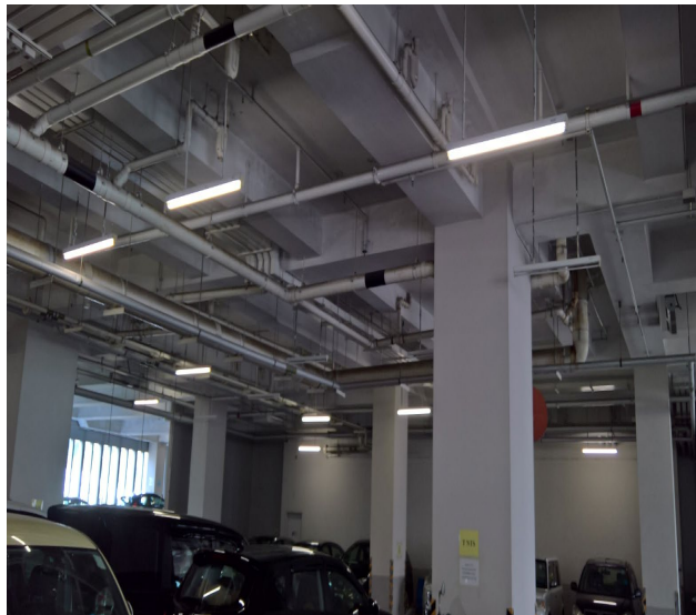
Photo A.19 Carpark lighting
