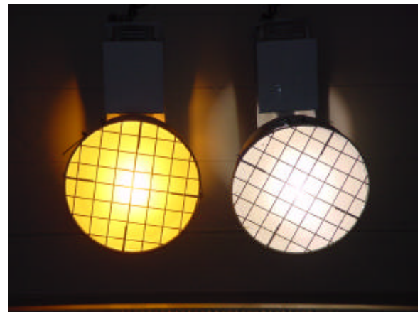
Fig. 2: Existing HID lamps and high-bay luminaires at KBIGH
