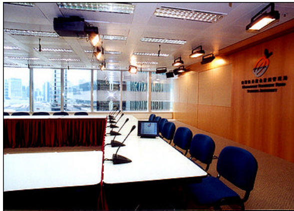
Figure 8 – A typical IR SI installation in a conference room
