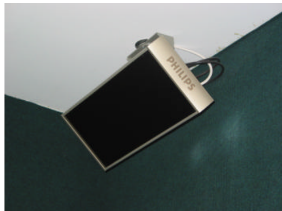
Figure 7 – A typical IR radiator used for SI system in a lecture hall
