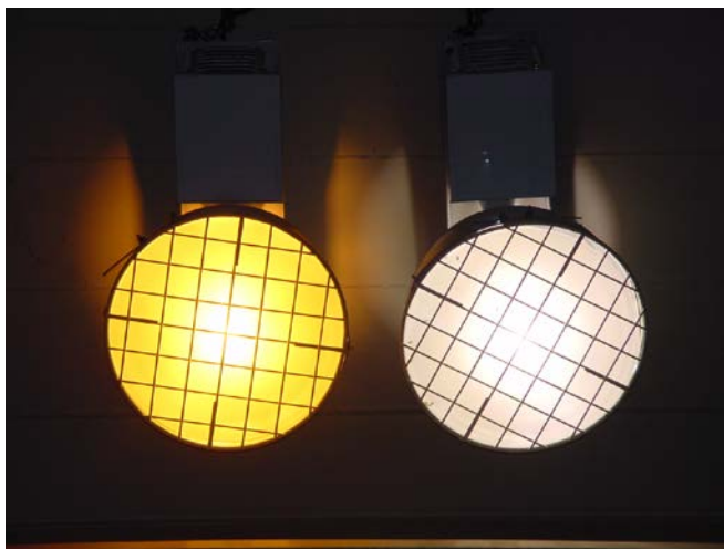
Fig. 3: Existing HID lamps and high-bay luminaires at EKT Indoor game Hall
