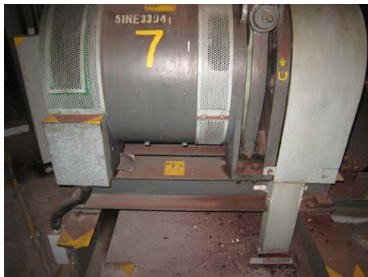
Photo 3 – No damage found on the main drive.
