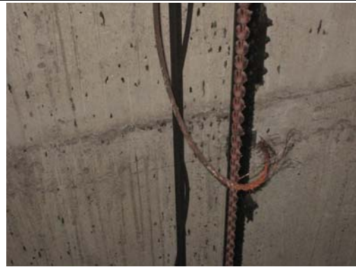
Photo 2 – Broken rope hanging inside the lift shaft.
