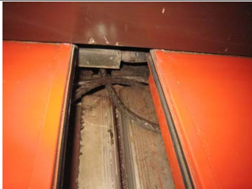
Photo 1 – Broken rope hanging on the lift car door at 24/F.
