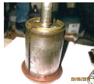
Figure 9: Condition of right brake plunger (No lubricant was found)
