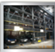
Mechanised Vehicle Parking System
