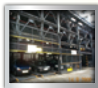
Mechanised vehicle parking system
