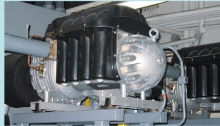
一座附有可變速壓縮機的450噸冷凍機能達到平均效率每噸0.324千瓦 A 450-ton chiller fitted with variable speed centrifugal compressors can achieve an average efficiency of 0.324 kW/ton
