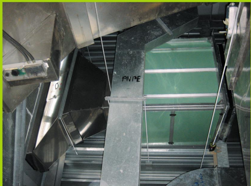
送風櫃加設了排氣風扇和排氣管 The AHU is fitted with additional exhaust fan and duct
