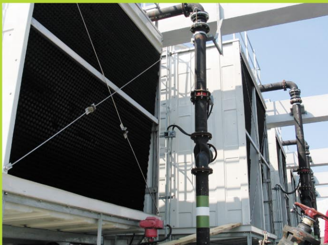
九龍紅磡香港理工大學李兆基樓 (冷卻塔散熱量：9,400 千瓦) Hong Kong Polytechnic University Lee Shau Kee Building at Hunghom, Kowloon (Heat Rejection Capacity: 9,400 kW)
