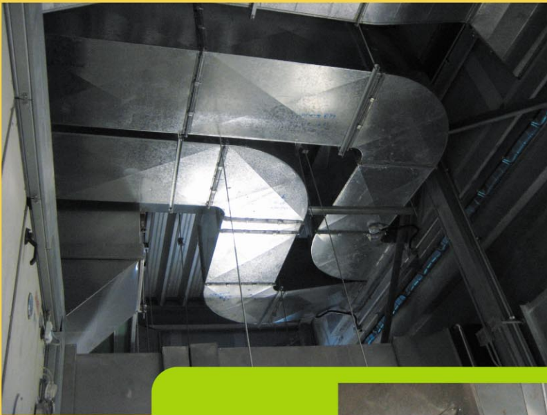
機電工程署能源效益事務處的送風櫃須加裝鮮風喉 Additional fresh air ducts are installed at the AHU in the EEO of the EMSD HQS
