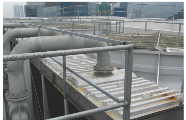
北角廉政公署總部 (製冷量：約1,500冷噸) Independent Commission Against Corruption Headquarters Building at North Point (Cooling Capacity: about 1,500 TR)
